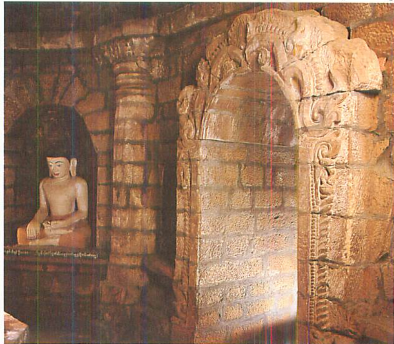
118 Andaw-thein. Inner passage, entrance to the western cross passage with ornate surround. A half-column of Indian Saracenic derivation supports the superstructure. The obtrusive mortar is the result of recent restoration.
